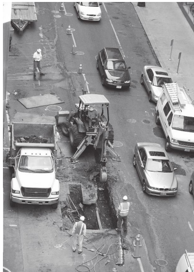
Disruption of traffic by utility repairs.
