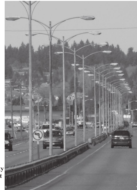
Street lighting - generally all paved surfaces in cities are lit every night, including all roads, parking lots, and parking structures.
