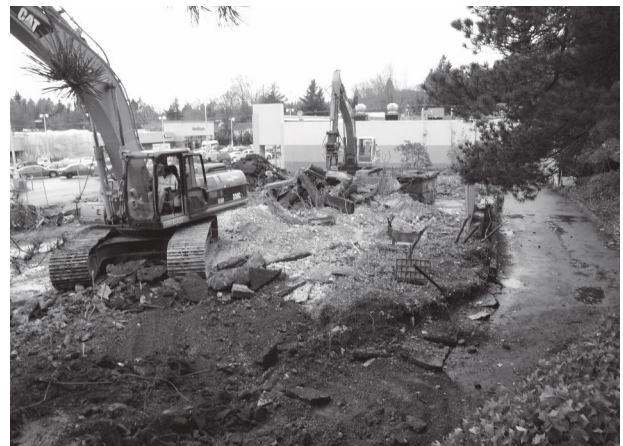
Premature demolition of a viable building, which was replaced by a parking lot.
