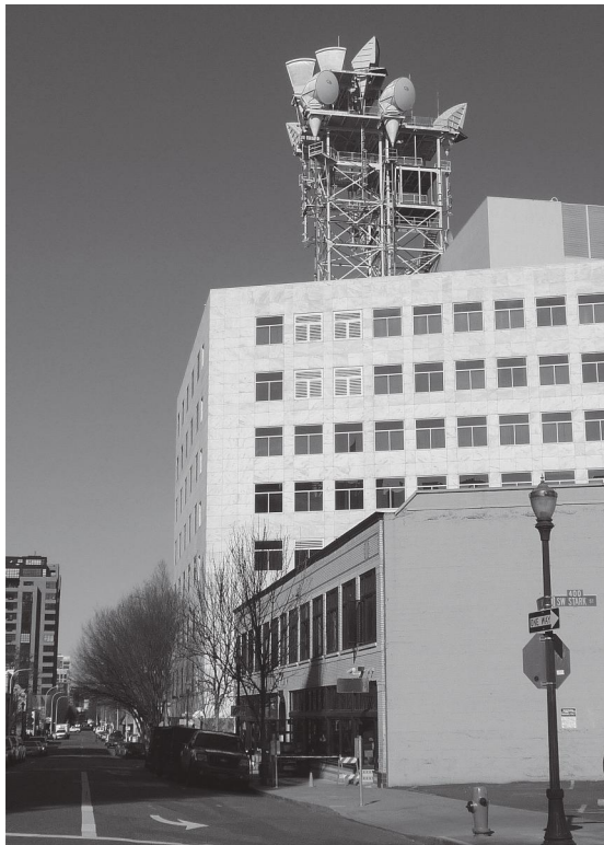
Communications array on top of a building.
