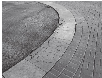
Automobile infrastructures are deteriorating all the time. The elements and wear and tear take their toll. Maintenance and up keep are a continuous chore for city, county, and state governments, and even for private citizens in regard to driveways and garages.
